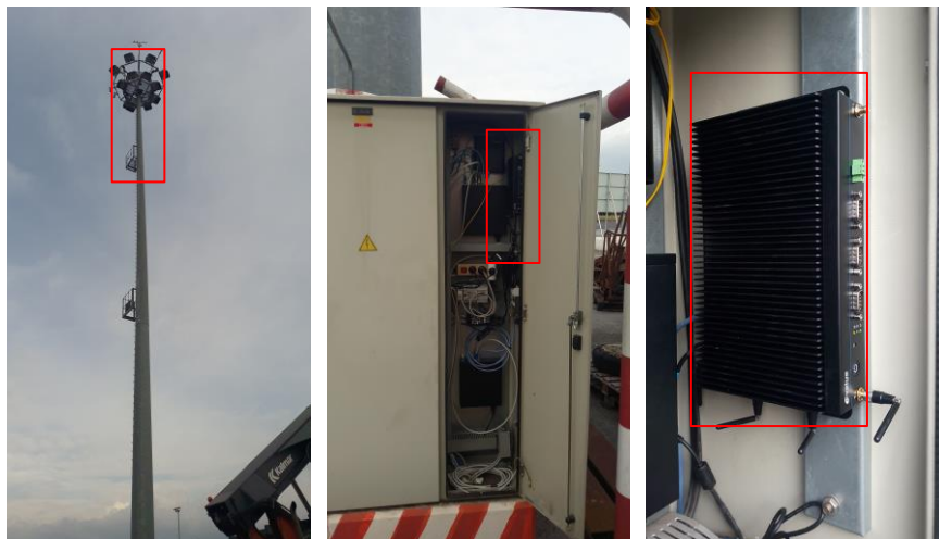
Figure 115: LL Koper - Light tower with deployed UHD camera (figure on the left), power shelter (figure on the middle) with deployed 5G GW (figure on the right).
