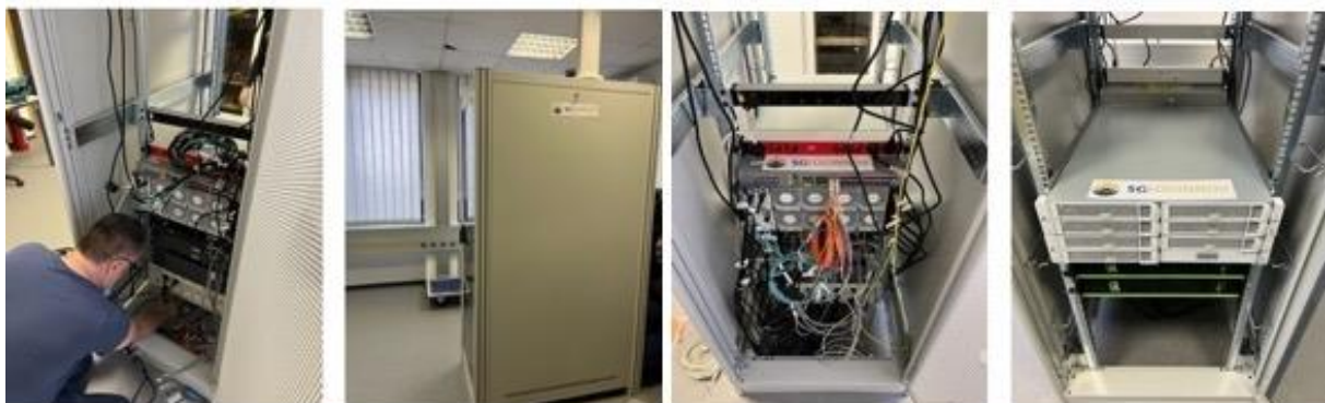
Figure 83: LL Koper – 5G NSA core network (SGW and PGW element) in Port of Koper cloud facility.
