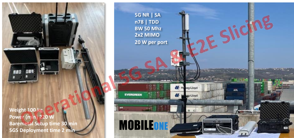
Figure 108: LL Koper - Private 5G System testing in Luka Koper/Port of Koper (April 2022).
