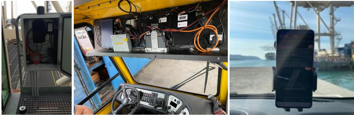
Figure 86: LL Koper - qMON Agent deployment for stationary and drive testing of the 5G NSA mobile network – (Left) 5G IoT GW on STS Crane, (Middle) 5G IoT GW on Terberg truck, (Right) Samsung S21 on port van.
