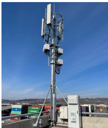
Figure 84: LL Koper – 5G NSA RAN deployed in Port of Koper.
