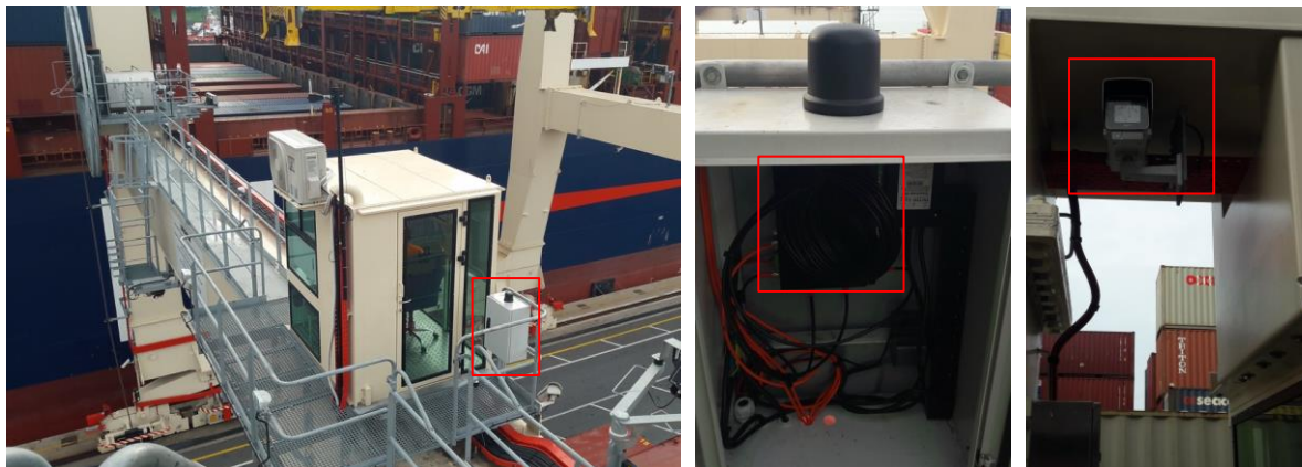
Figure 114: LL Koper - Deployment of the shelter on the STS crane (figure on the left) with Industrial 5G GW inside (figure on the middle) and connected UHD camera (figure on the right).
