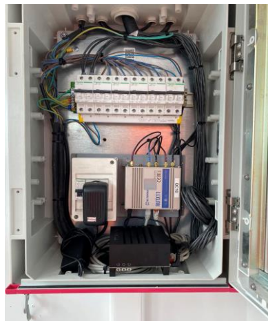
Figure 20: 5G modem and IoT node inside the cockpit of the crane
